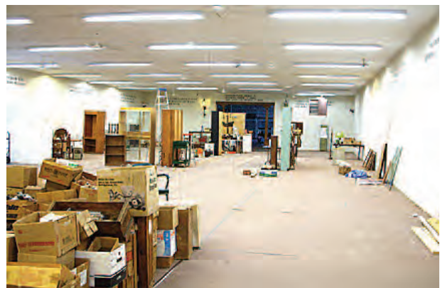
A portion of the new museum building. With the antique dealers gone, Ron Roche's crew will soon be demolishing various internal partitions to make way for new construction.
